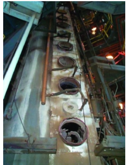
3. Modernizing. In addition to replacing Gibbons Creek's fuel piping, the emissions-reduction project team improved primary air control by installing modern airflow instrumentation and replacing the original damper drives and several dampers. Courtesy: Burns & McDonnell
