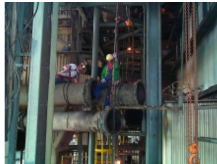
2. Downsizing. More than 4,000 feet of 26-inch-diameter fuel piping was replaced with 24-inch pipe in only 21 days. Courtesy: Burns & McDonnell
