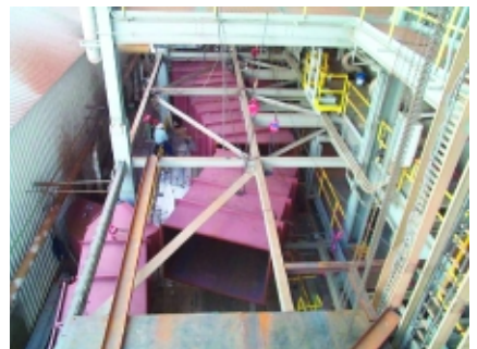
5. New ductwork. The TLN3 system installation required the addition of ductwork, which was routed through existing structural members without restricting access to any wall blowers. Four new windboxes were placed about 30 feet above the primary windbox. Courtesy: Burns & McDonnell
