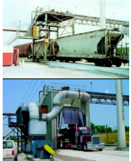
6. Dusting solution. At this plant, severe dusting from a combination railcar/open truck loadout facility handling powdered bulk materials was causing safety problems (top). The solution was to design better seals for the belt conveyors and loading spout and an enclosure to surround the facility and shield it from the wind. Slotted dust collection hoods with pickup hoods were ducted to a dust collector unit and fan mounted outside (bottom). Courtesy: CDG Engineers
