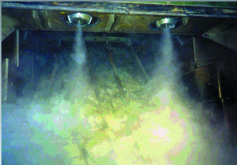
Dry fog is expanded externally and away from nozzles at this feeder-to-conveyor transfer point to control PRB coal dust, and thus reduce explosion hazards
