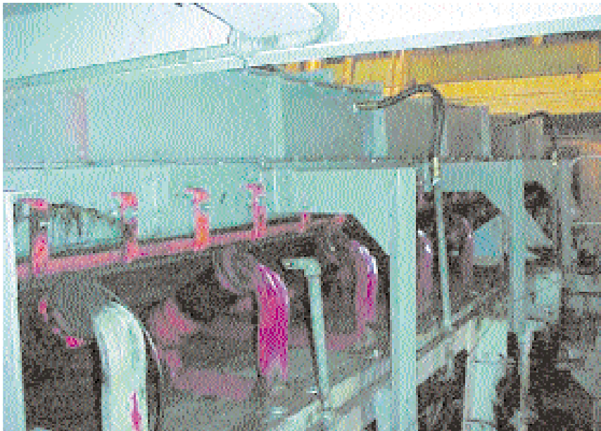
6. Good housekeeping is crucial to preventing coal-dust fires and explosions
